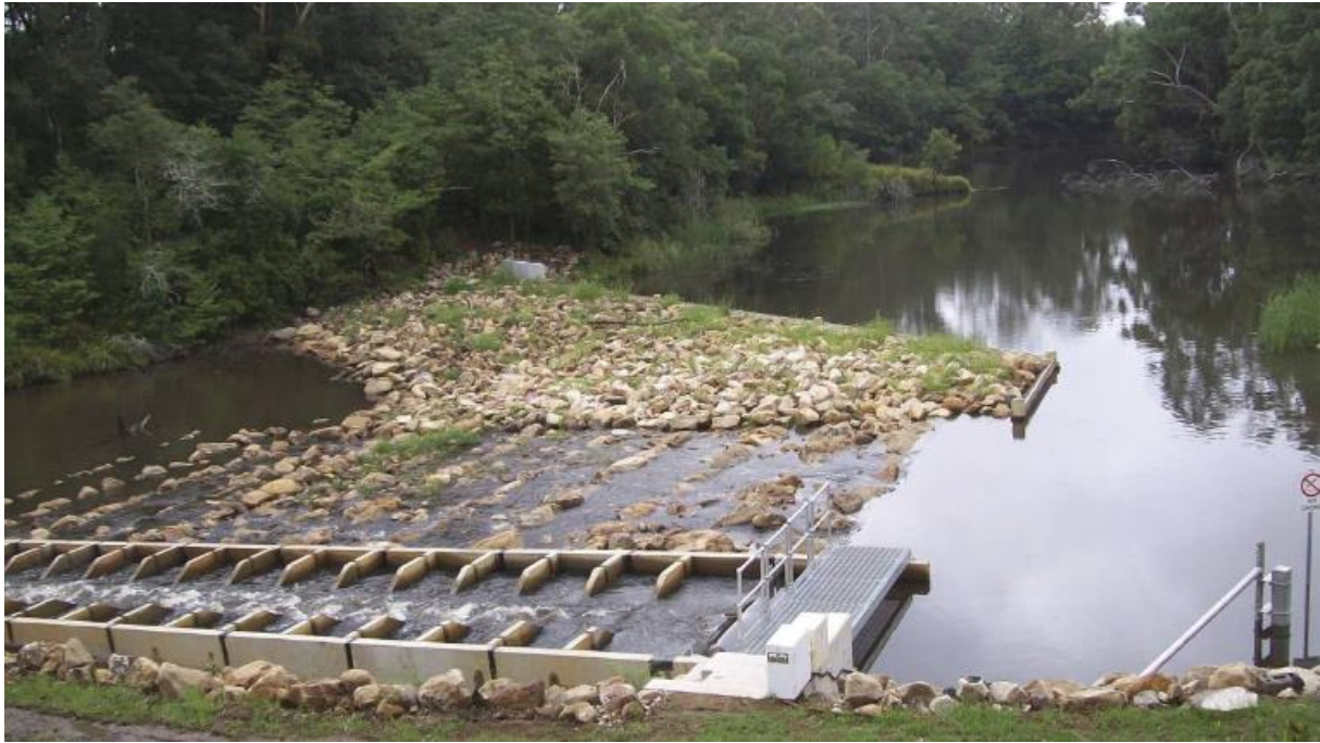
Figure 3.2 Wyong River Weir and fishway (reprinted from Newcastle Herald published on 17 October 2016)
