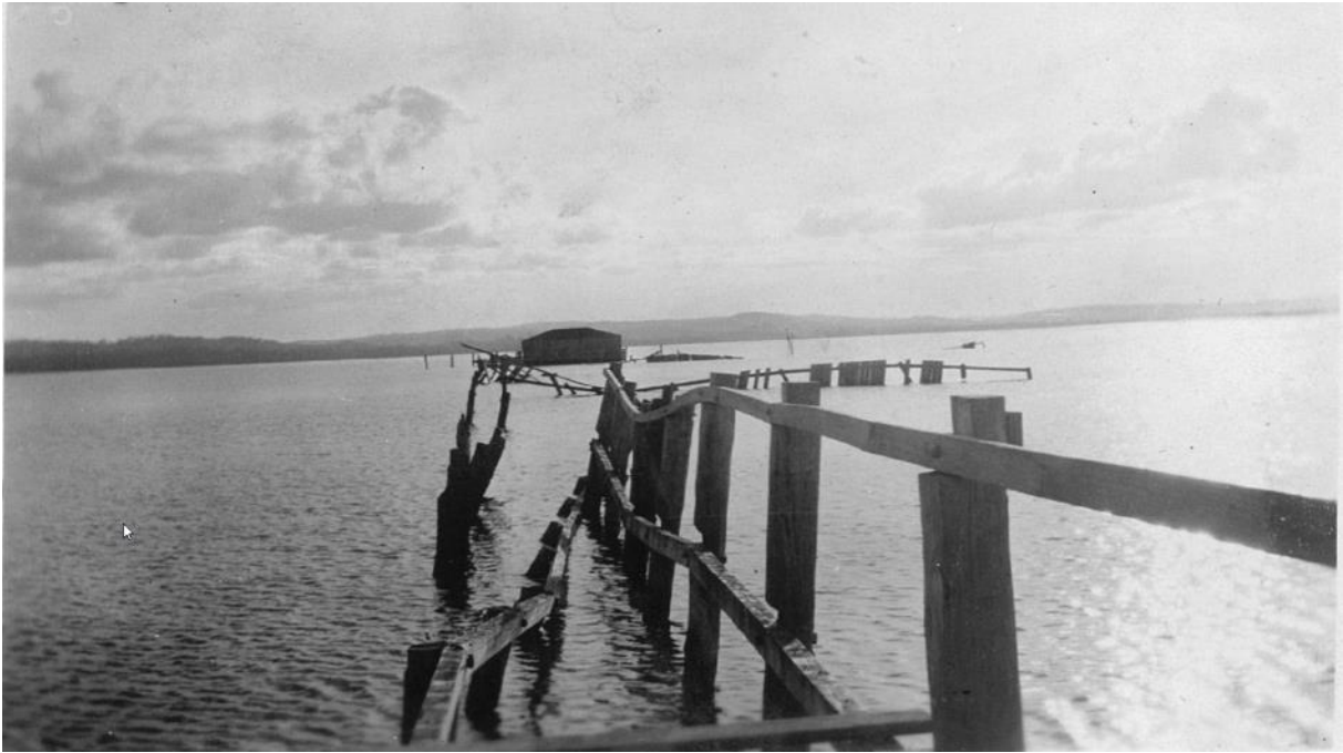
Figure 1.2 Damages to the original Long Jetty (built 1914 by William Henry Price) following flooding in Easter 1927. Courtesy of Central Coast Council
